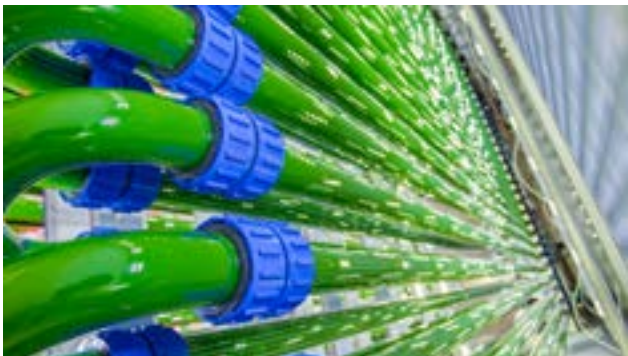
Figure 4. A fully enclosed photobioreactor cultivation system under perfect climate and contamination control at Algalif's site in Reykjanesbaer, Iceland.
